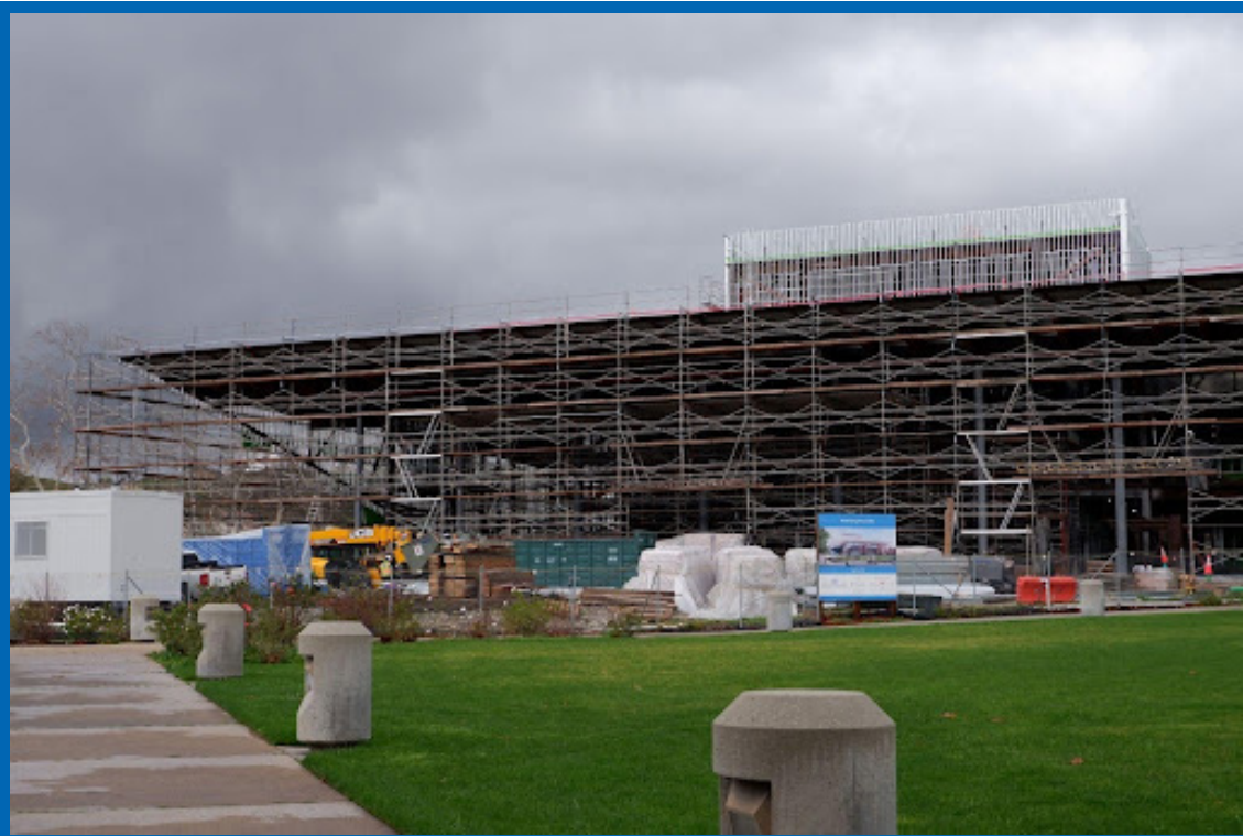
The construction of the new Performing Arts Building Photo by Jocelyn Martinez-Lopez
