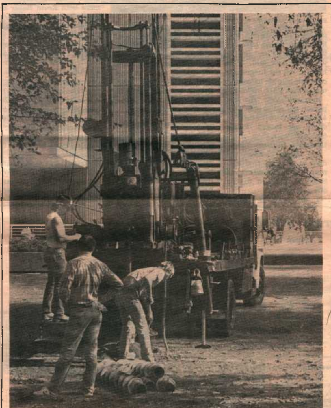
Construction workers use a drill to test soil strength for proposed buildings. The site shown is for the Pfau Library addition.
